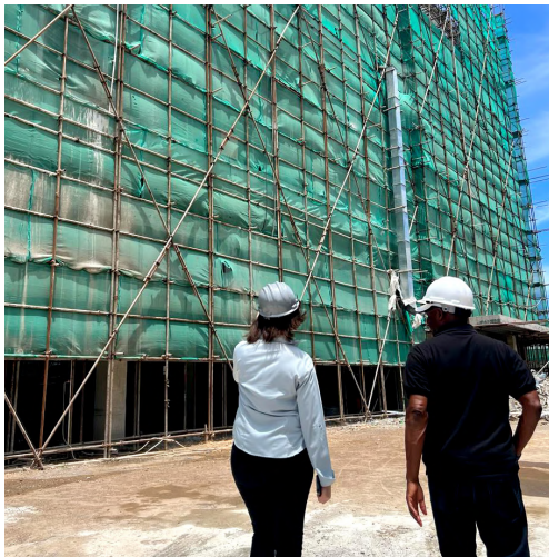
Chairman and CEO, Melanie Subratie leads Minister of Industry, Investment and Commerce, Senator, the Honourable Aubyn Hill on a tour of the construction site of the new Unit 1.
